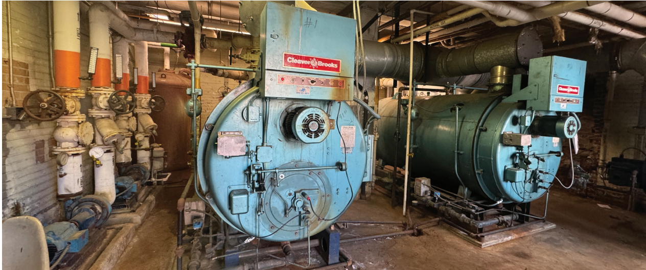
Hickman Central Plant
