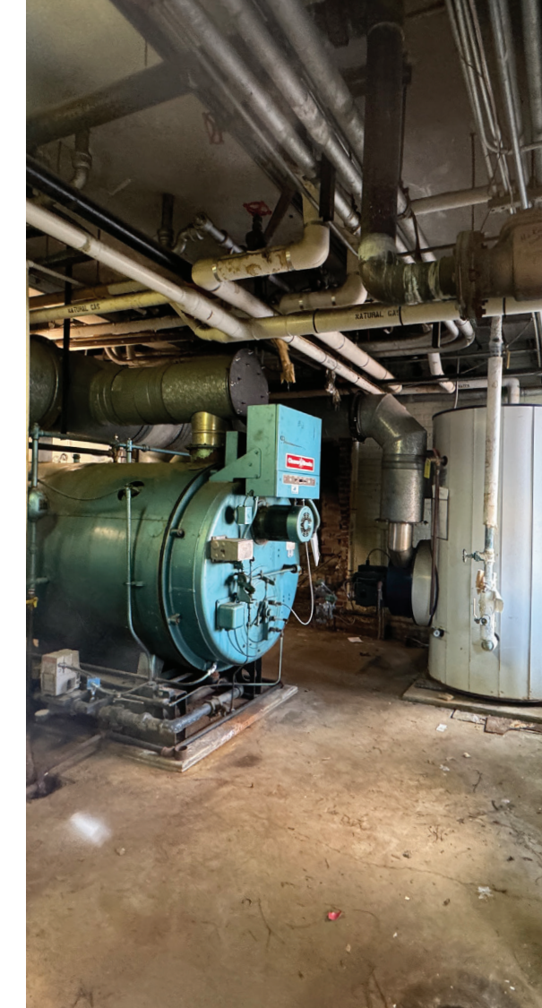
Hickman Central Plant
